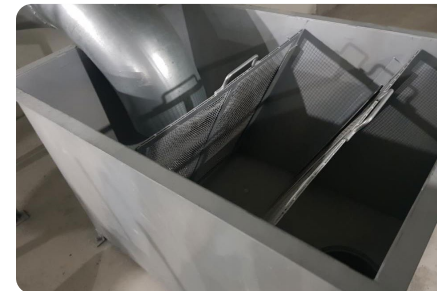
Rainwater tank – collection screen
