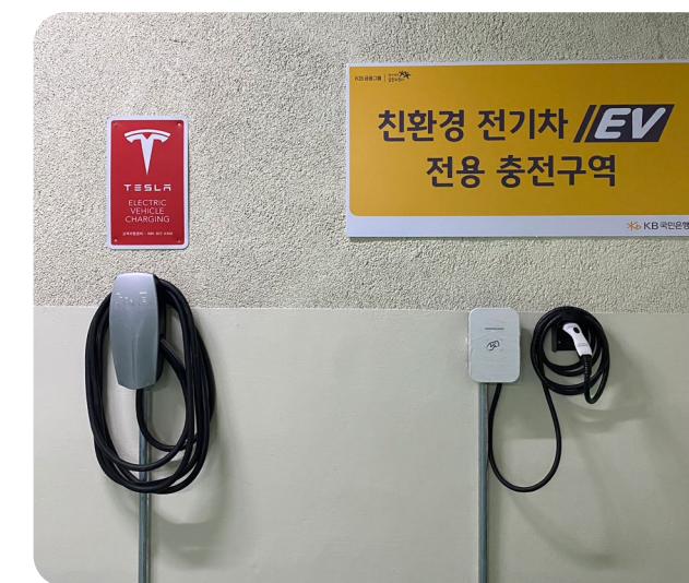
EV Charging Station
