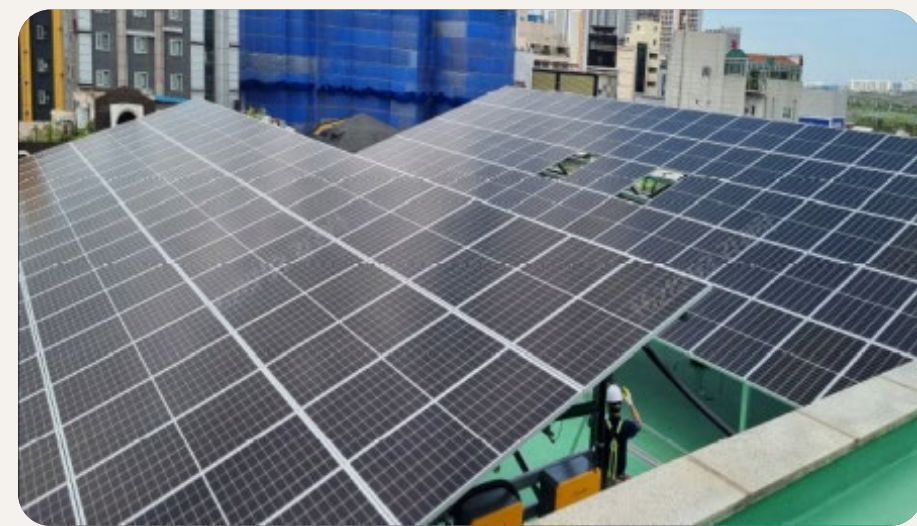
Solar power generation facility at Pyeongtaek Central Finance Center
