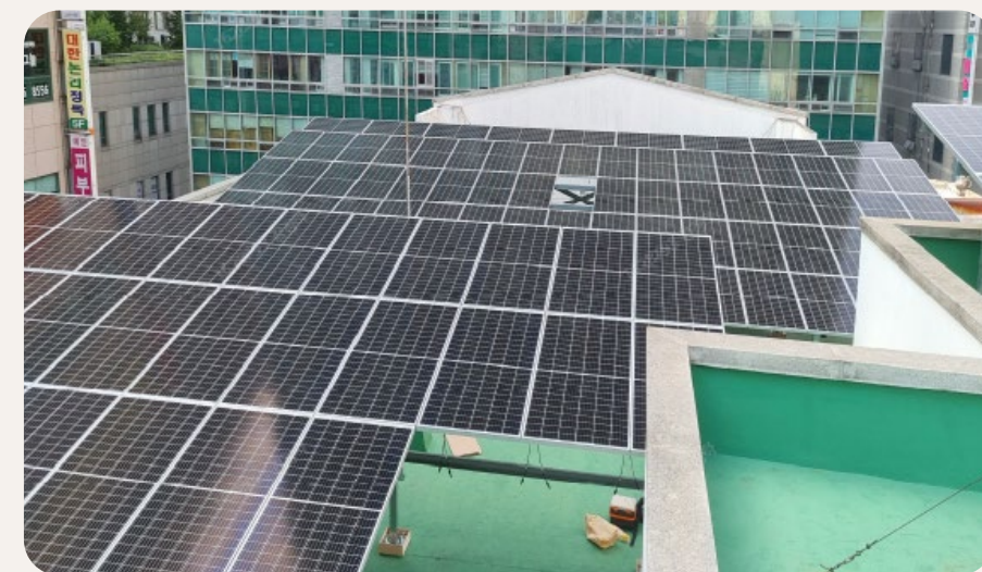
Solar power generation facility at Mokdong PB Center
